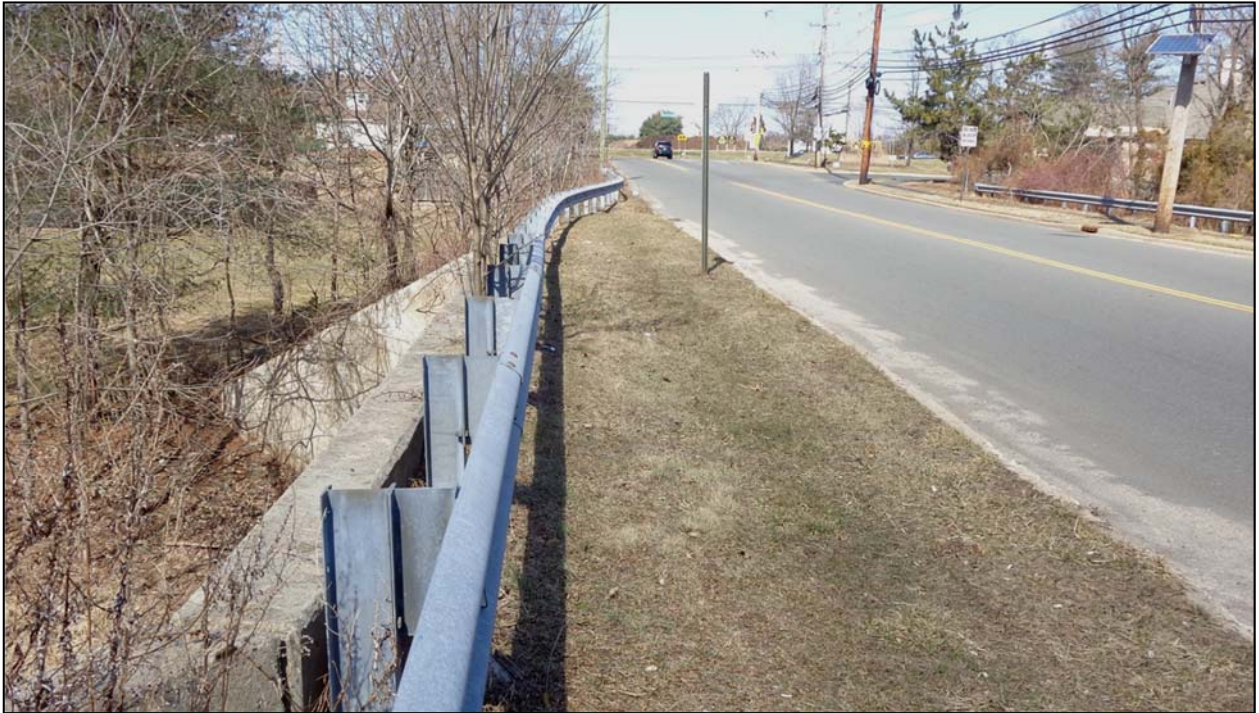
Photo No. 1: View looking west along New Brunswick Road from bridge towards Cedar Grove Lane.
