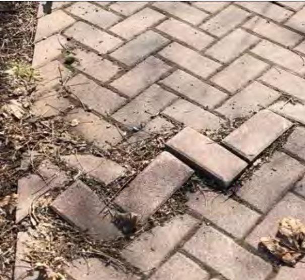
Brick paver sidewalks need to be reset and repaired along corridor
