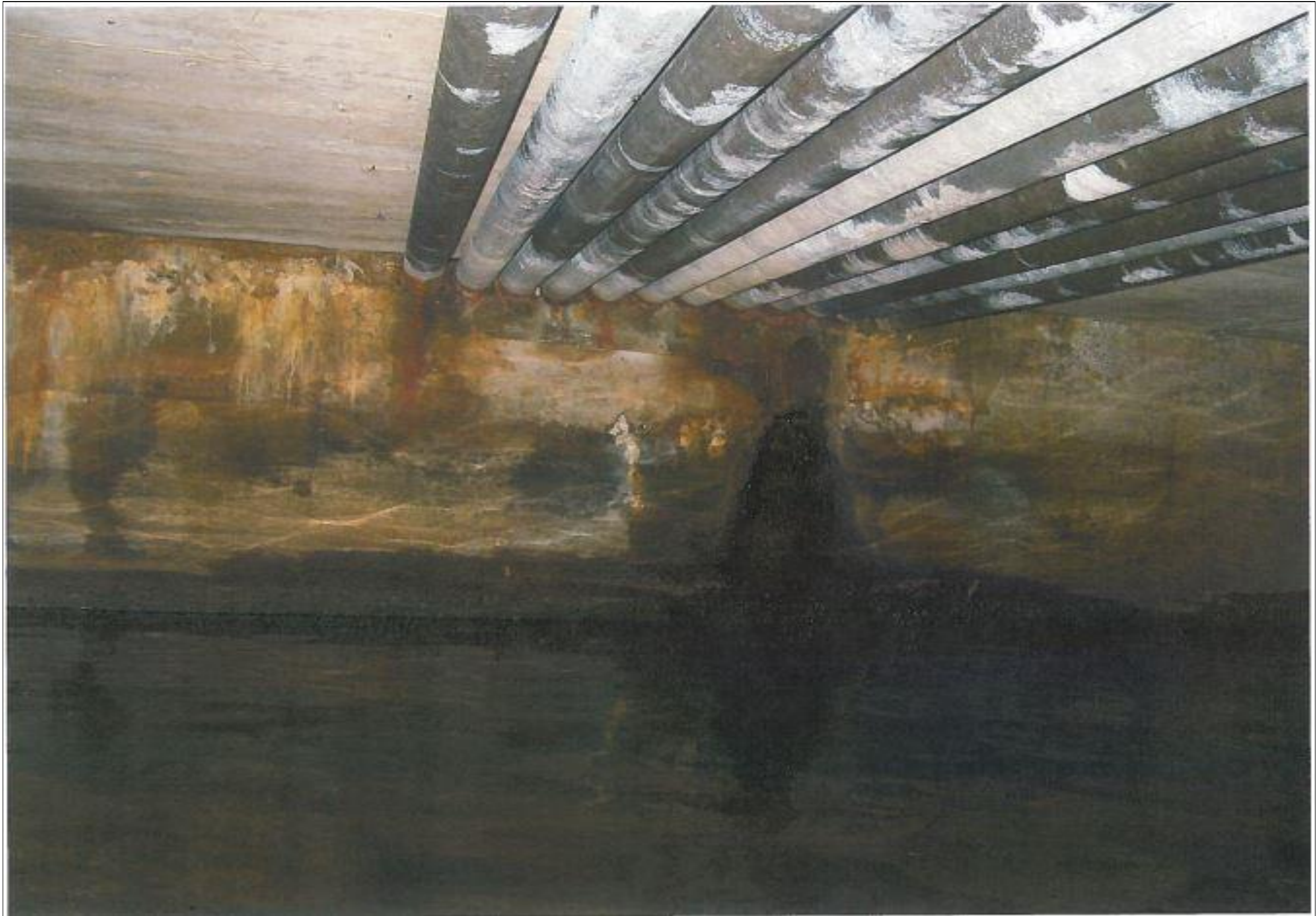
PHOTO 5 M1019 SOMERSET STREET: LOOKING NORTH AT TELEPHONE CONDUITS
