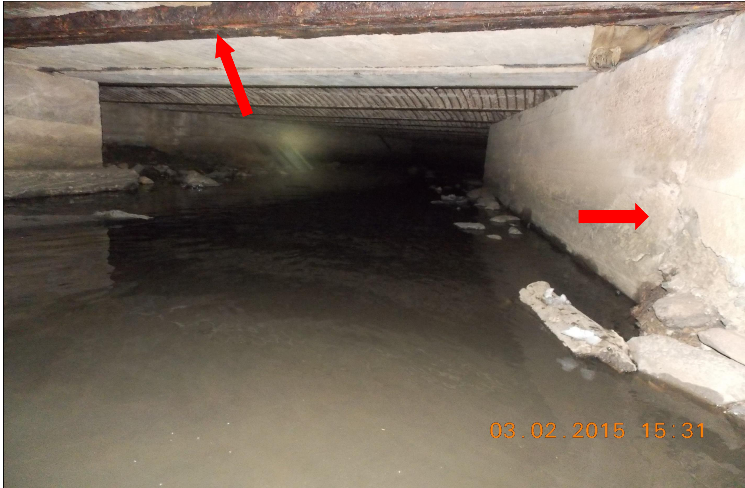
PHOTO 6 M1019 SOMERSET STREET: LOOKING WEST AT ADJACENT DOWNSTREAM STRUCTURE. IT ALSO EXHIBITED SEVERELY CORRODED STRINGER AND SPALLED ABUTMENT
